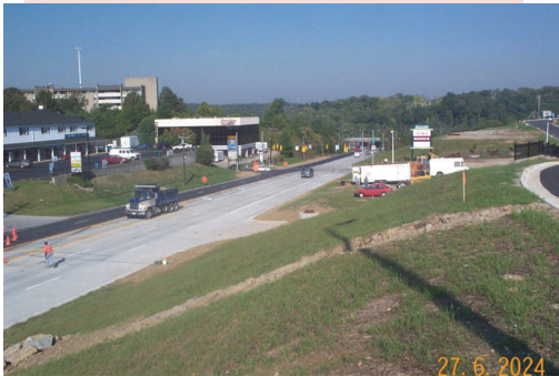
The project on Harrison Avenue at Rybolt and I-74 took 30 days to complete
