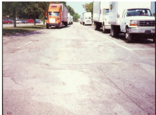
Deterioration of the pavement caused ODOT to update this rest stop using concrete.
