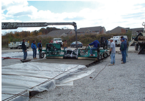
The stone base enhances the water holding capacity and curing with visqueen insures success.
