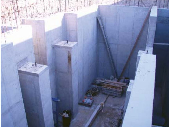
The average machine foundation project Swederski Concrete performs utilizes 1,000 yds. of concrete and 30 tons of reinforcing steel.
